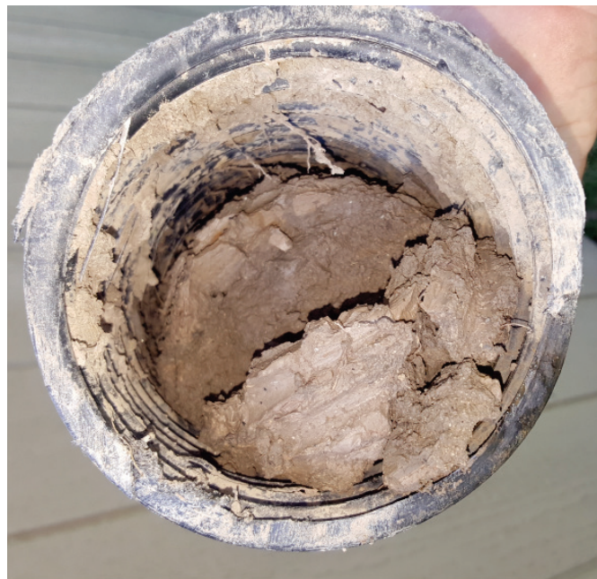
Figure 2d: Foundation Drainage Pipe Blockage
