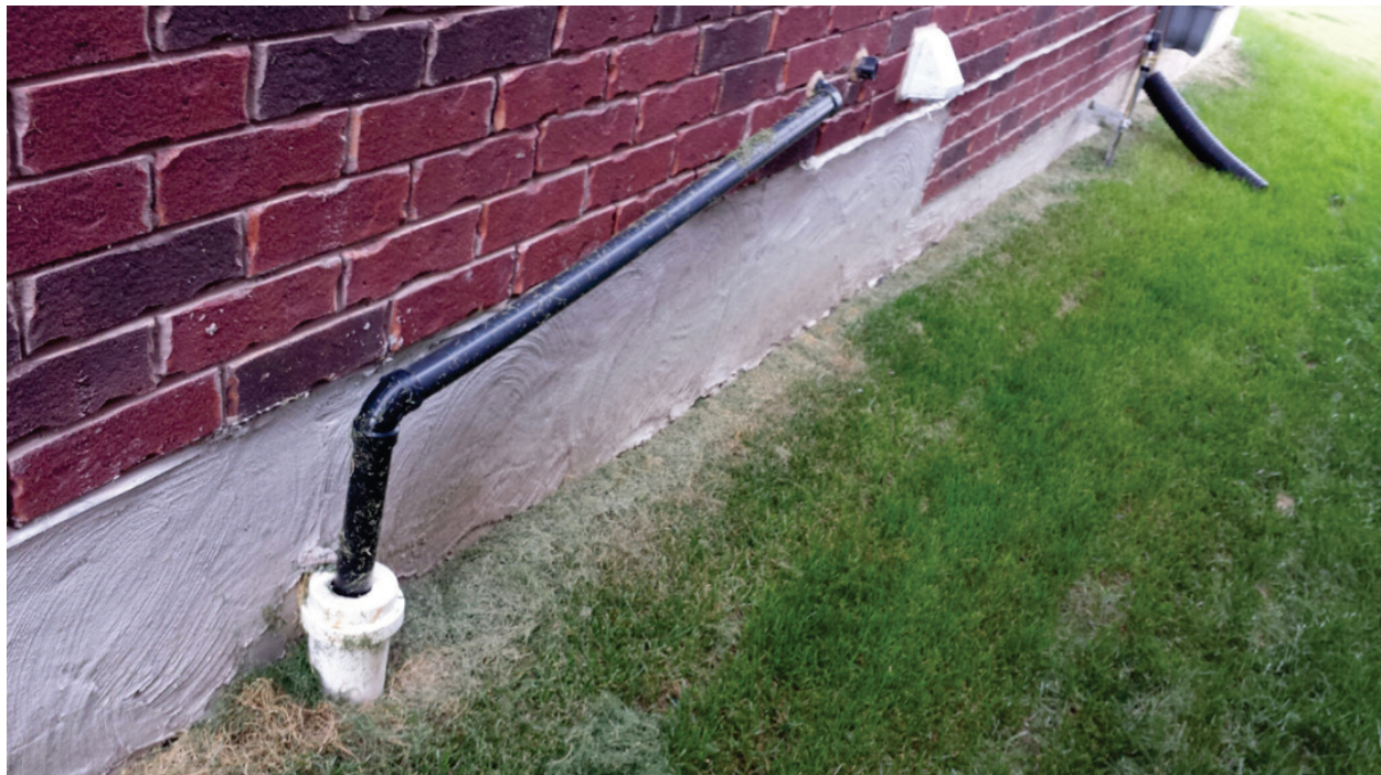
Figure 3l: Sump Pump Discharge Pipe Entering a Downpipe (Collingwood, Ontario)
